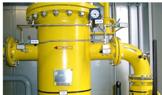
Fig. 2. Biomethane piping and measurement equipment in the grid connection station, Germany.
